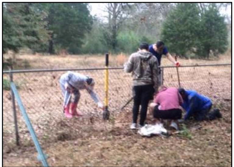
Re-installing the perimeter fence for the Zahn cemetery was a major task for Nate's crew.
